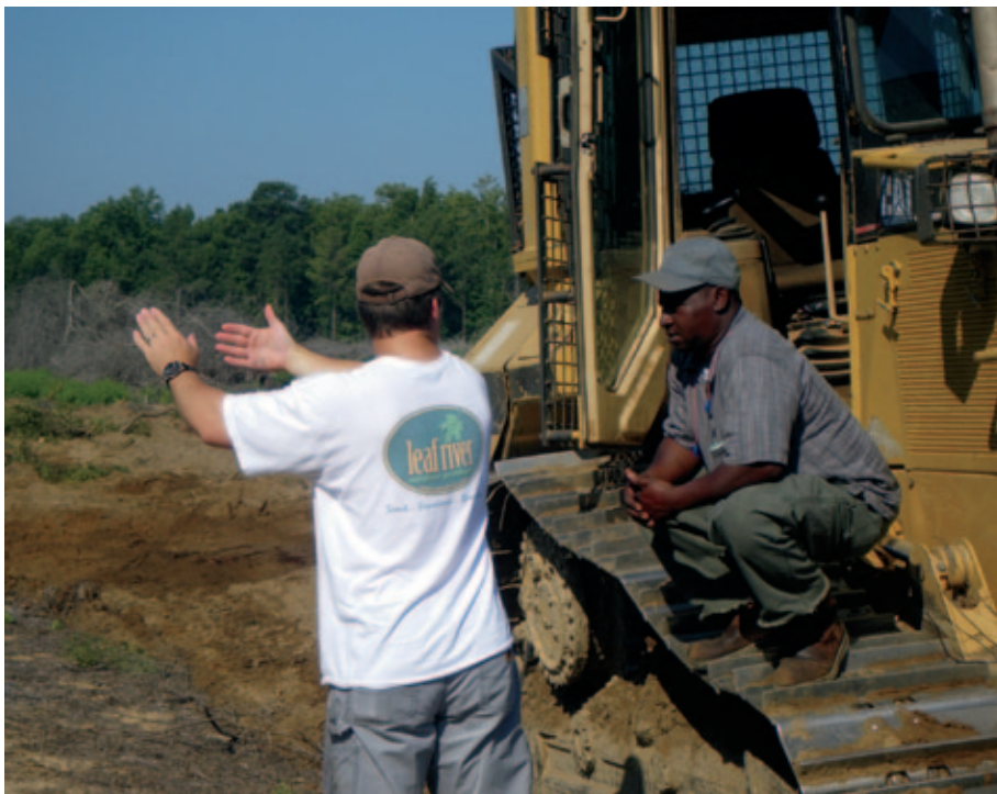
Road maintenance is a never ending project for a landowner. Winter is a great time to identify areas that need work.
