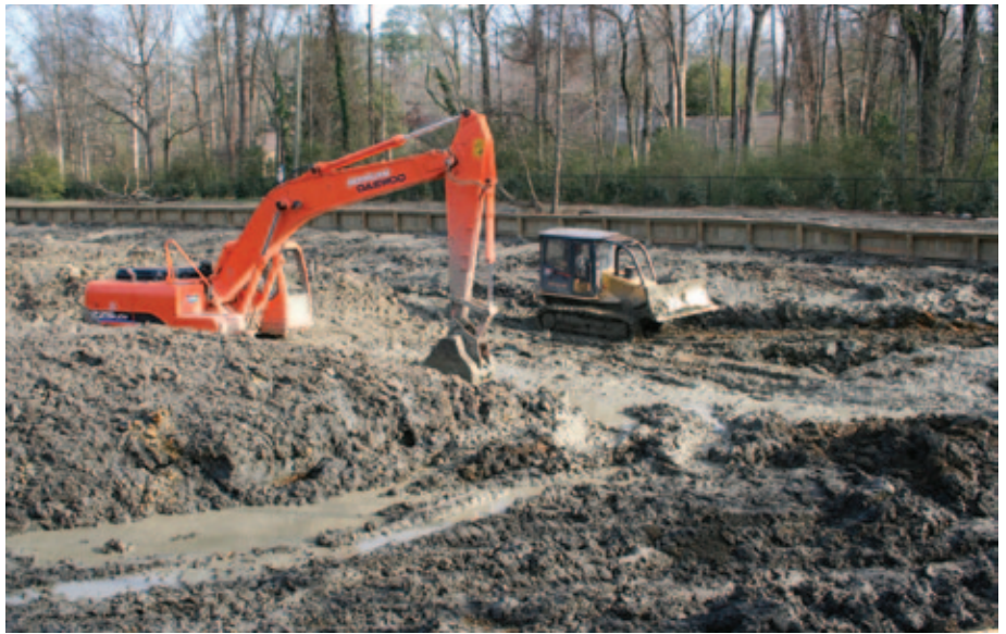
Heavy equipment such as an excavator and a bulldozer should be used to correctly build the lake of your dreams.
