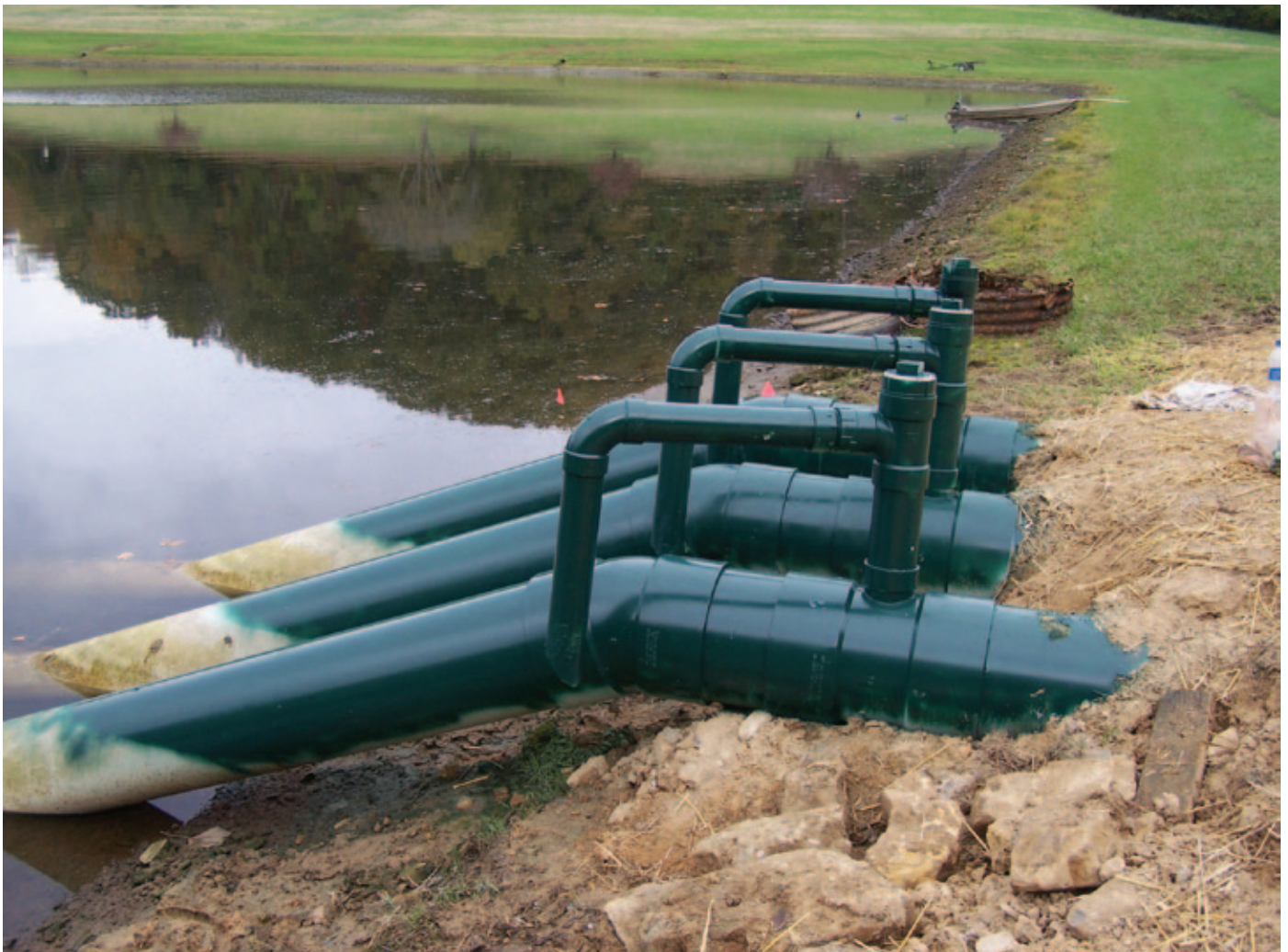
Siphon systems, such as this multiple pipe system, work great as the main water control structure.
