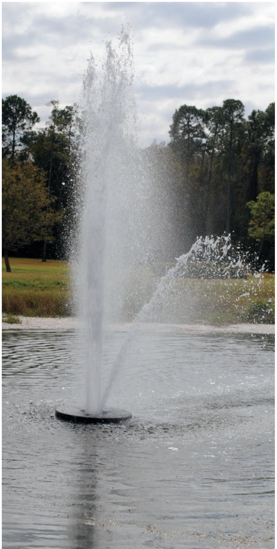
This fountain is clogged (notice how the spray pattern is not uniform) and needs to be cleaned. It can be and should be cleaned any season, as long as you can tolerate the air and water temperatures to perform the work.
