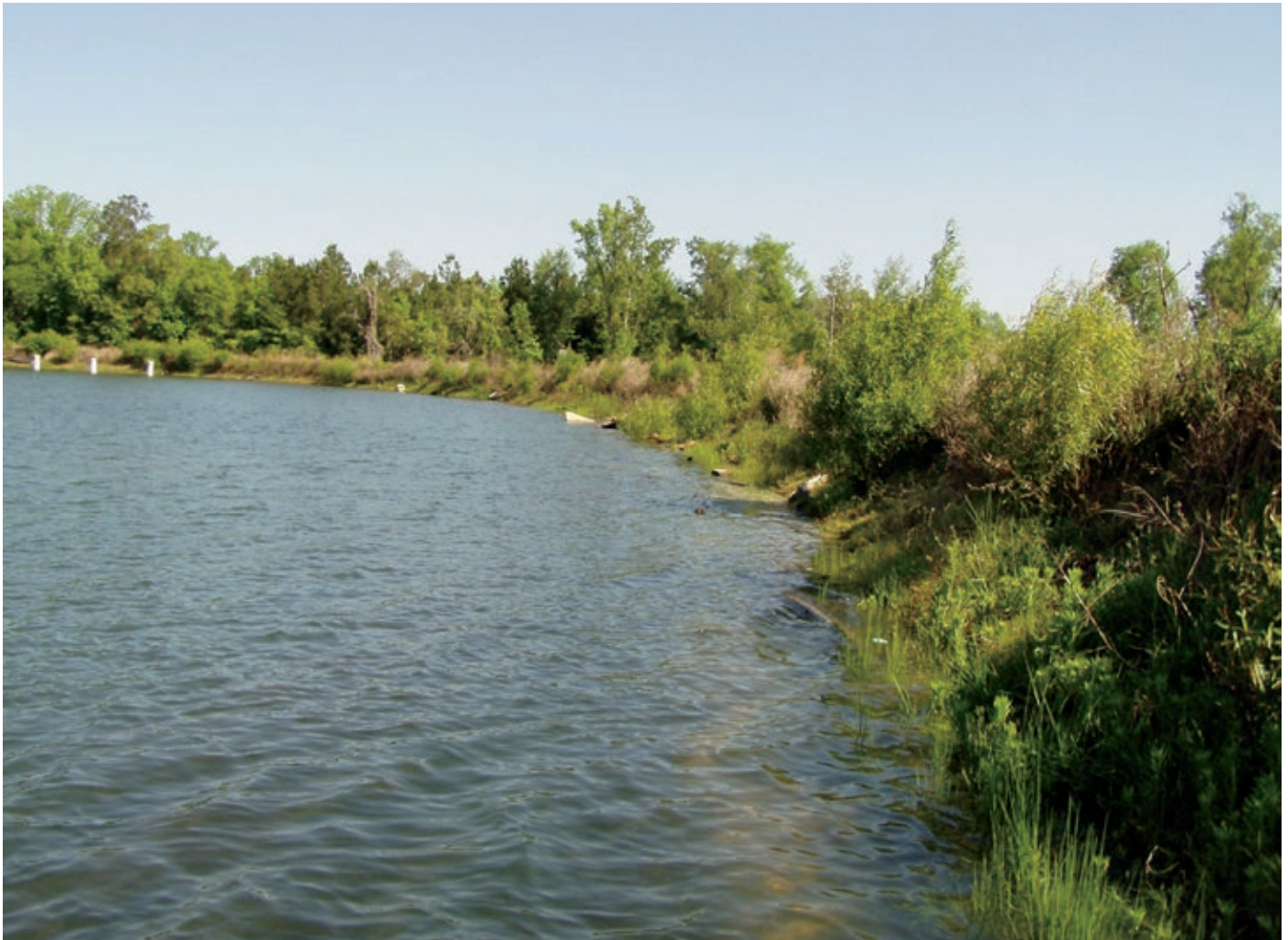
This lake dam has multiple species of trees growing on it. Treating with herbicide and cutting down or mowing of unwanted hardwood and pines should be done annually so they do not get out of control.
