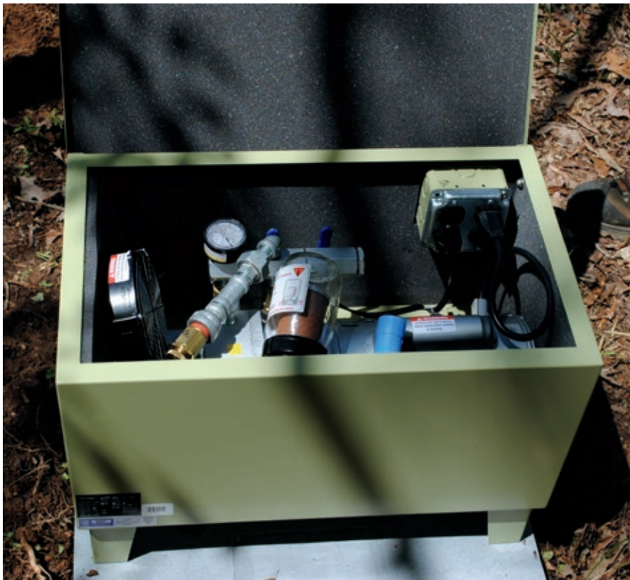
Checking the proper operation of fountain and aeration systems every six months helps prolong the life of the pump and other parts.
