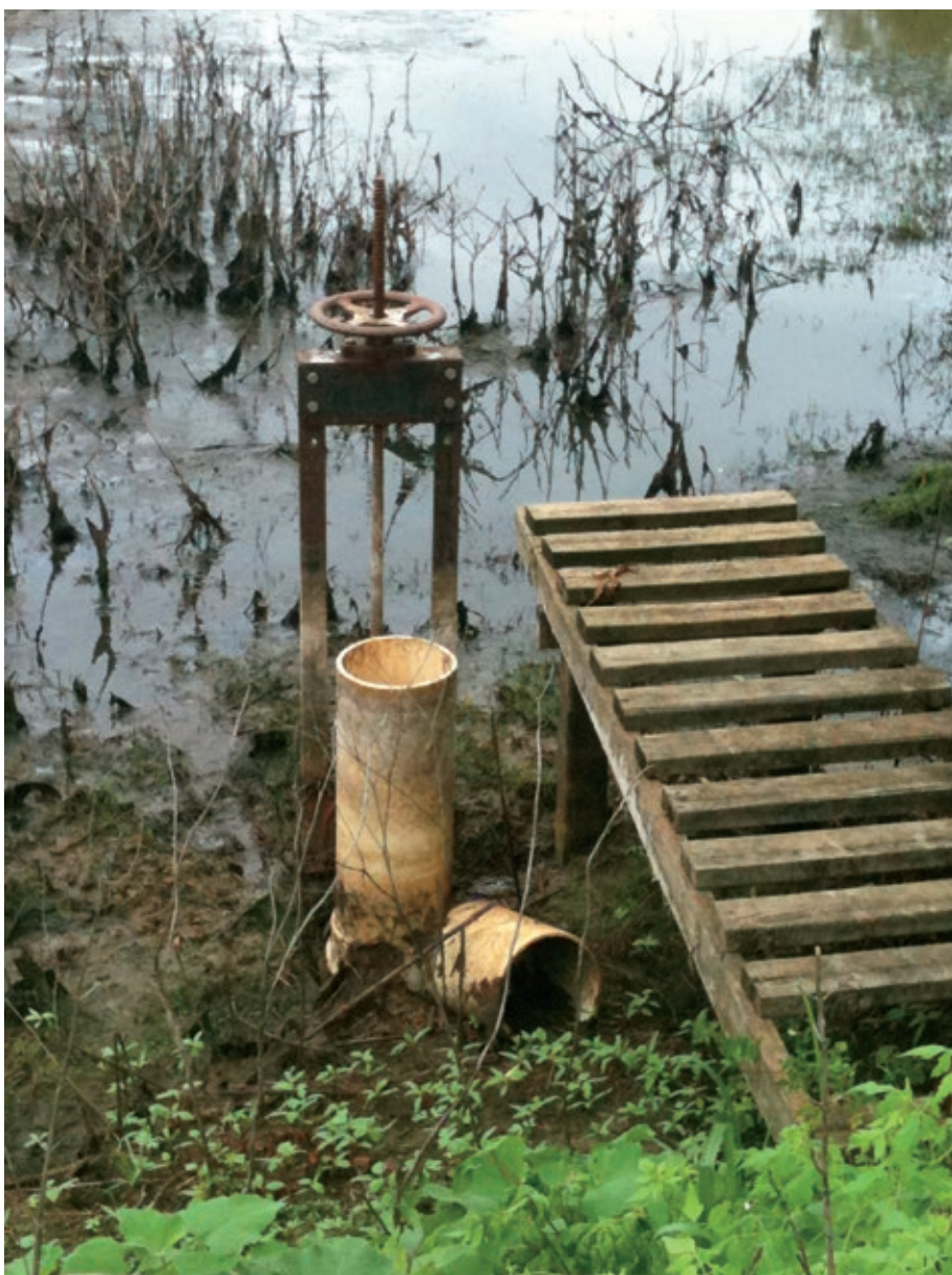
Early summer, which is often the driest period in the Southeast, is a good time to inspect and make repairs to water control structures.
