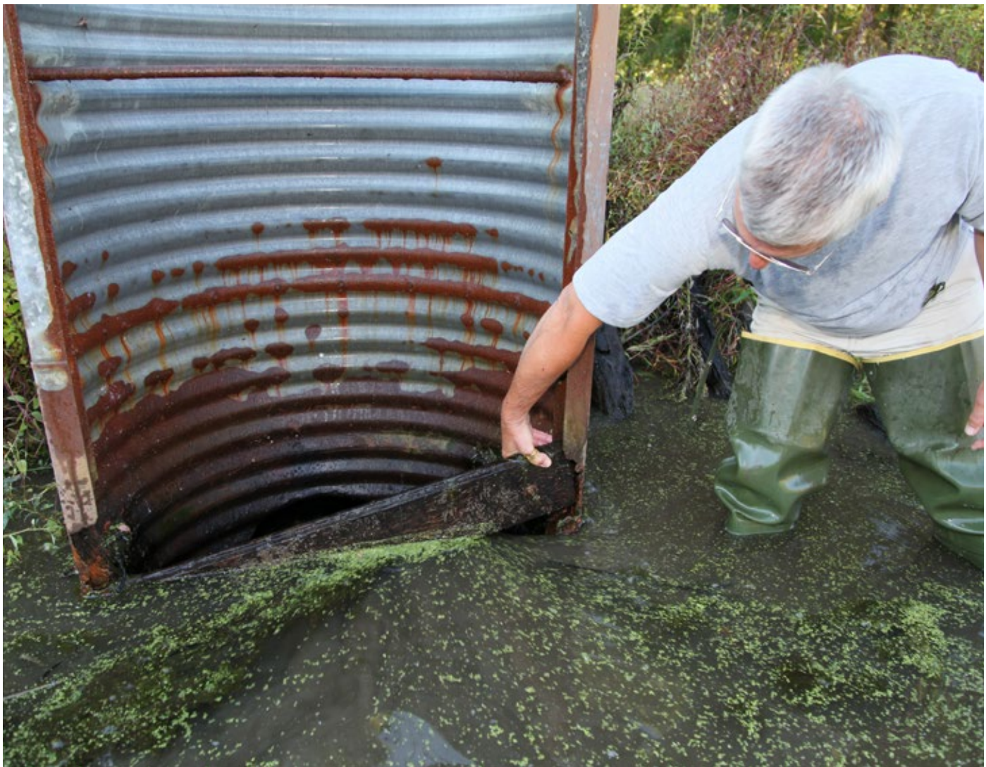
Early summer is a great time to check and repair water control structures.
