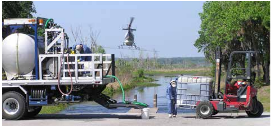
Once vegetation management techniques like this are employed the expense is very high. It is recommended to stay on top of vegetation management on big water.
