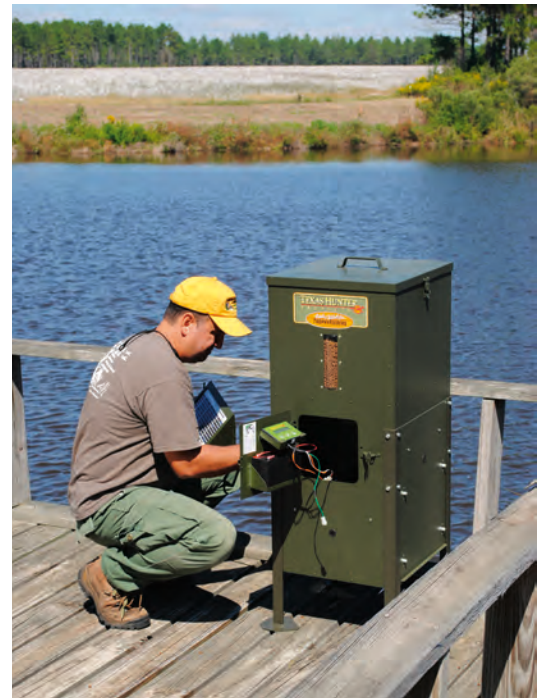
Winterizing in late fall and servicing in late winter keeps batteries fresh and everything working smoothly during the upcoming year.
